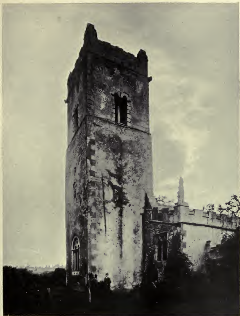
ST. MARGARET'S CHURCH TOWER, MARTON (BEFORE RESTORATION).
